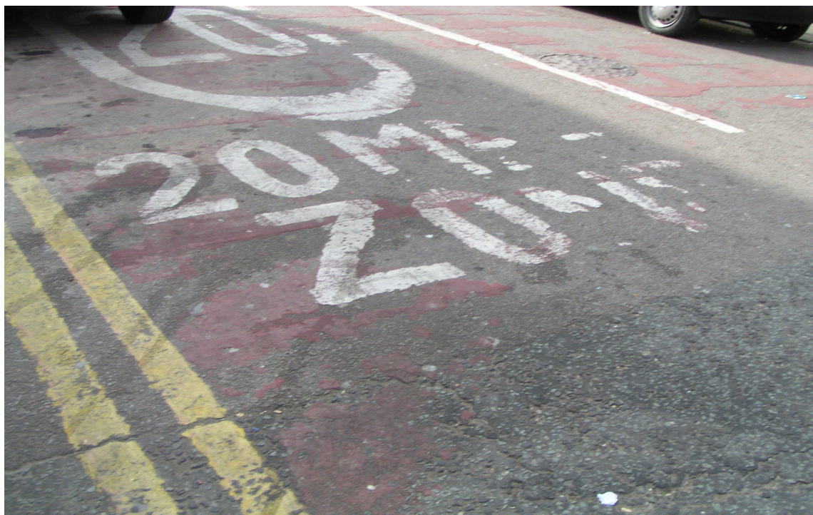
Deteriorating surface markings on 20mph signs should be repainted
